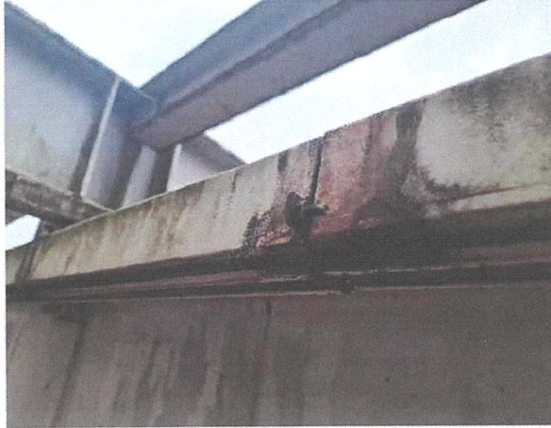
Hoist Crane Boiler IDF 2 AB 10 Ton, Power supply, Other fault
